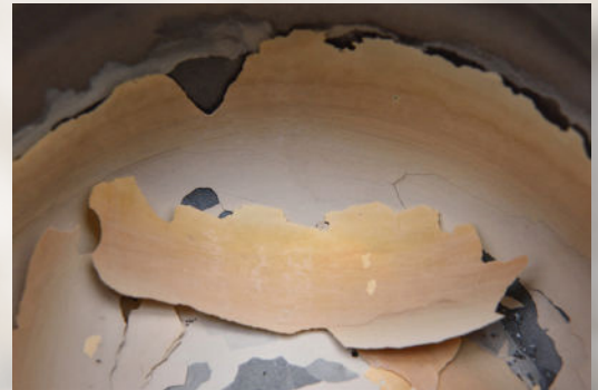
Water heater with scale and sediment buildup decreasing the efficiency, water pressure and lifespan of this water heater.
