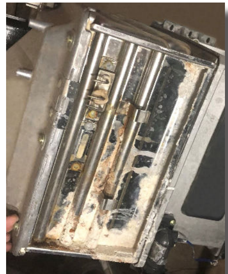
Lime scale buildup on a tankless water heater without ScaleRx ® protection in Phoenix, Arizona
