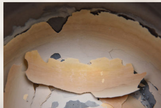
Water heater with scale and sediment buildup decreasing the efficiency, water pressure and lifespan of this water heater.
